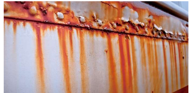
Figure 1. Failure of protective coating in preventing corrosion on ferrous metal.
